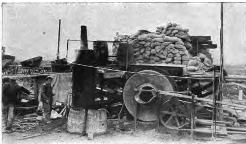
FIG. 2.—HEATING MIXING WATER BY EXHAUST STEAM. Note water tank at top of mixer.
